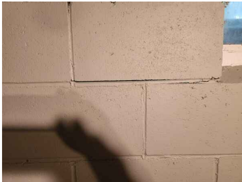
Same Wall as Step Crack with distortion
