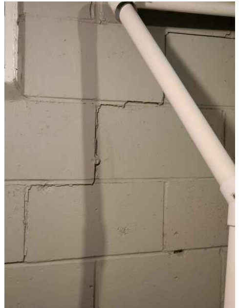
Step Crack with Distortion
