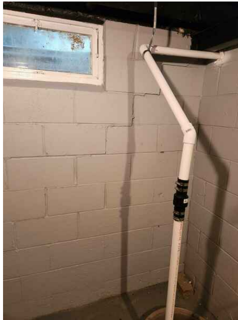
Step Crack with distortion
